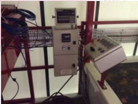
Computerised control panel in the 16 m 3 mixing plant
