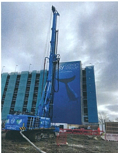
Supplying secant piling rigs with a special pre-blended Material giving strength from 0.7-1.00 Mpa @ 28 days
