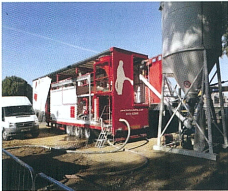
16 m 3 batching plant and silo.
