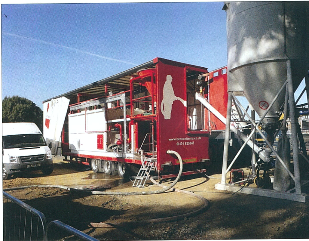
Photograph Above. Site set up of a 16m 3 bentonite batching mixing unit producing up to 300+m 3 /day
